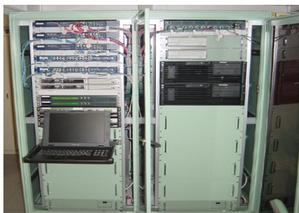
Fig. 1 Network Server Room
