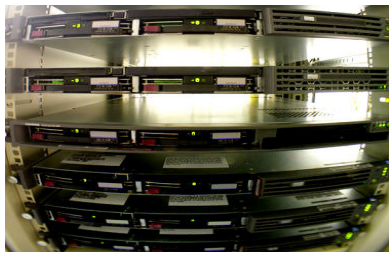
Fig. 4 All 16 Network Servers
